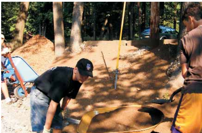
Members of Boy Scout Troop 73 of Westfield add topsoil and mulch to the border of the main parking lot.
