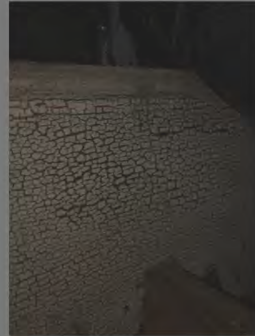
Fig. 2: A view of a board in the original opening access opening in the ceiling below the cupola. Note the shadow line on the top of this board and the manner in which the subsequent coats of green, red, and other layers do not fully cross that threshold. That shadow line is consistent
